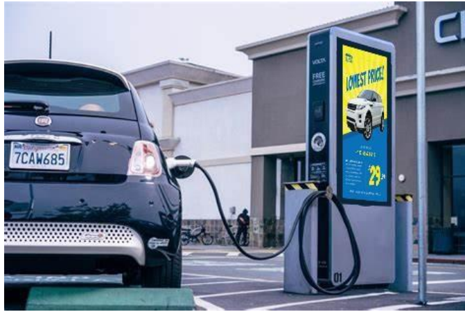
EV charging station
